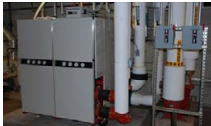
New chiller at Wade Hampton High School
