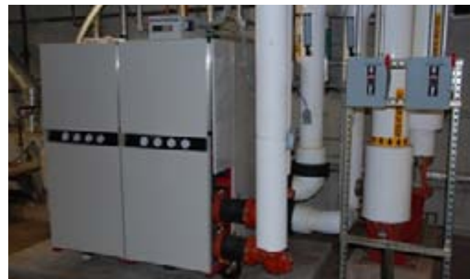
New chiller at Wade Hampton High School
